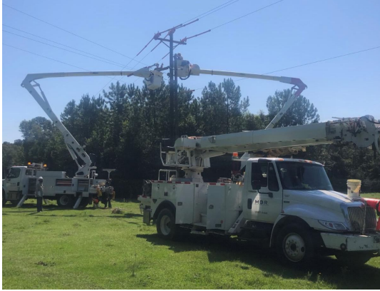
SR Connect contractors prepare poles in the Brewer pilot area before running fiber.
